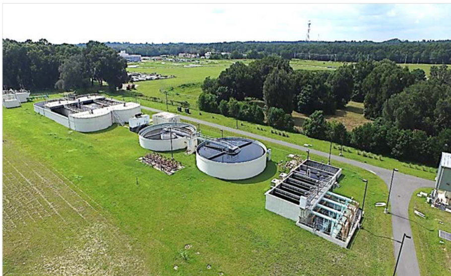
Aerial view of the City's Wastewater Treatment plant.
